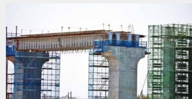
北陸新幹線の高架工事 Elevated structure works for the Hokuriku Shinkansen
