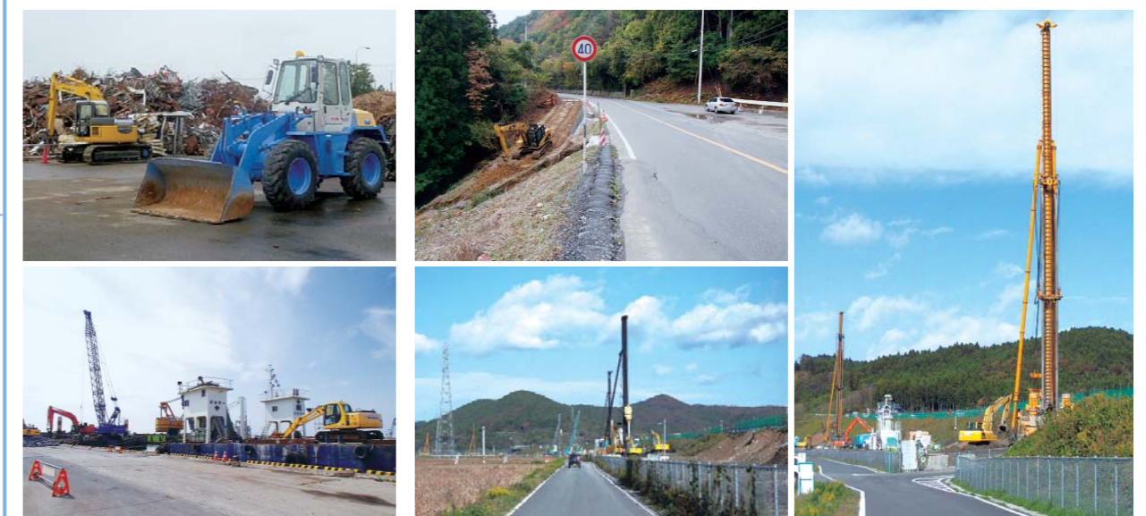
小名浜港(福島県いわき市:上)や石巻港(宮城県石巻市:下)など、港湾の復旧工事に使用される当社建機 Kanamoto's construction equipment is being utilized for port restoration works in places such as Onahama Port (Fukushima Prefecture, upper photo) and Ishinomaki Port (Miyagi Prefecture, lower photo)
