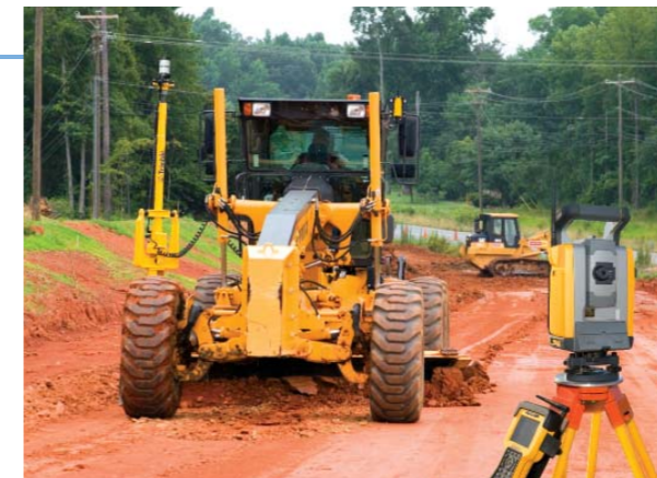
国土交通省が推進する情報化施工の現場 Site using information-aided construction technique promoted by the Ministry of Land, Infrastructure, Transport and Tourism
