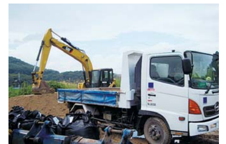
福島県飯館村で除染作業を行う当社の油圧ショベルとトラック Kanamoto hydraulic excavator and truck used for decontamination work in Iitate Village, Fukushima Prefecture.
